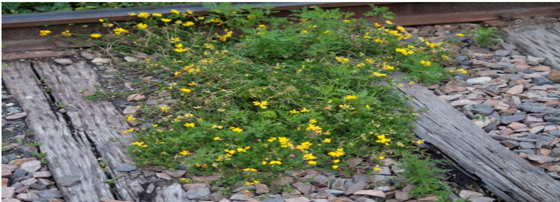
photo 7: Washington Cty RR. Do these cross ties comply with CFR 49 Sec 213.109 above?
